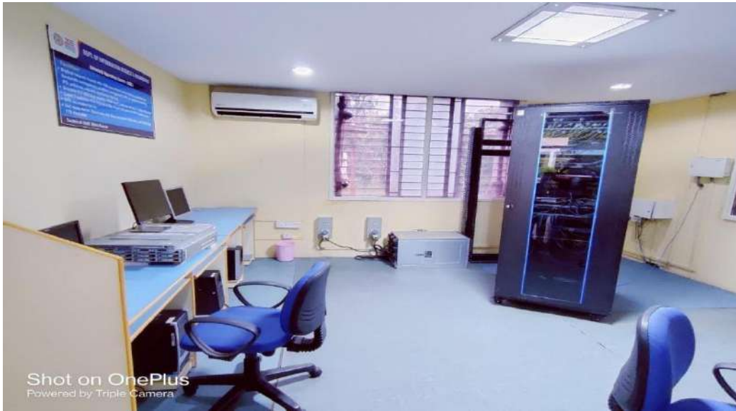
Network Operating Center
